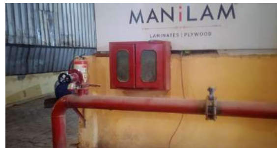
Fire safety system installed at our factory
